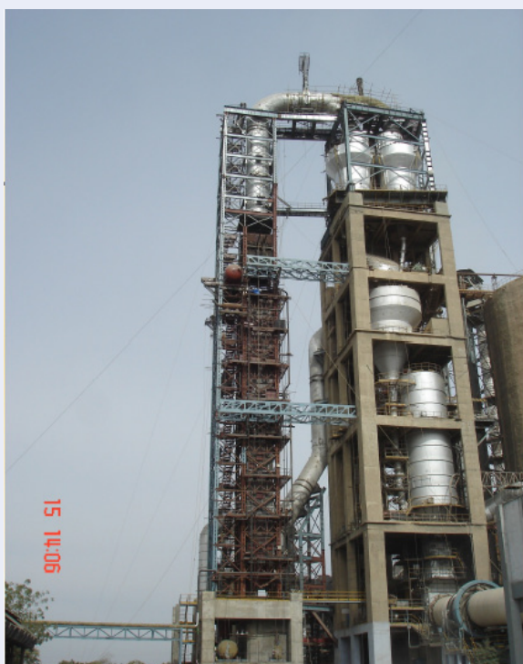
Cement plant waste heat recovery is increasingly of interest. (Courtesy: Transparent Energy Systems)
