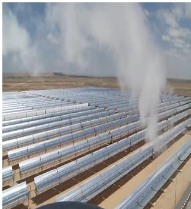
A Successful PPP - The Concentrated Solar Power Project in Ouarzazate Morocco (World Bank Photo).
